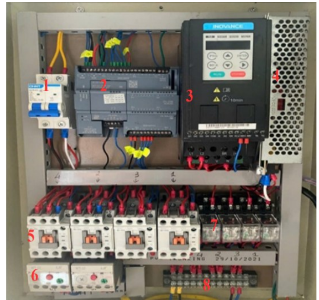
Fig. 6. Interior of the electrical cabinet: (1) Miniature Circuit Breaker (MCB), (2) Siemens S7-1200 PLC, (3) INOVANCE Variable Frequency Drive, (4) Power supply module, (5) Contactors (K1–K4), (6) Thermal overload relays (OL1–OL4), (7) Control relays (RL1–RL4), and (8) Terminal blocks
